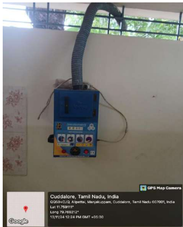
Incinerator in Ladies Toilet to Dispose Sanitary Wastes
