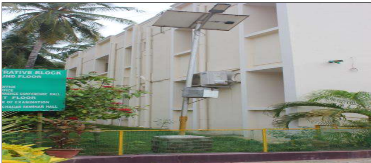
Street Lights Power Generated By Solar Energy
